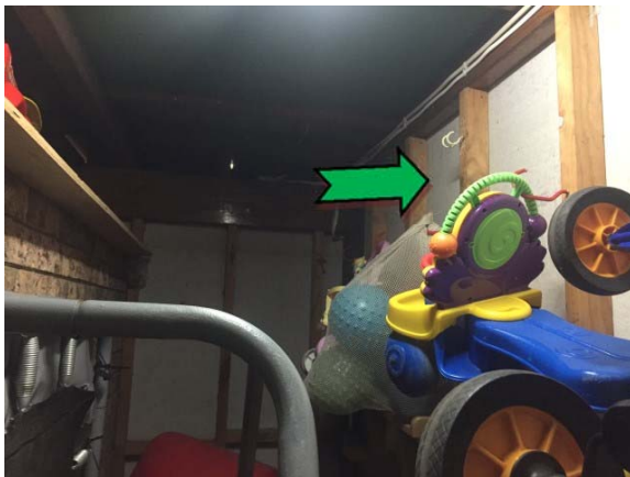
Photo 3. Interior, north store room, throughout, internal walls – non asbestos-containing fibre cement sheeting.
