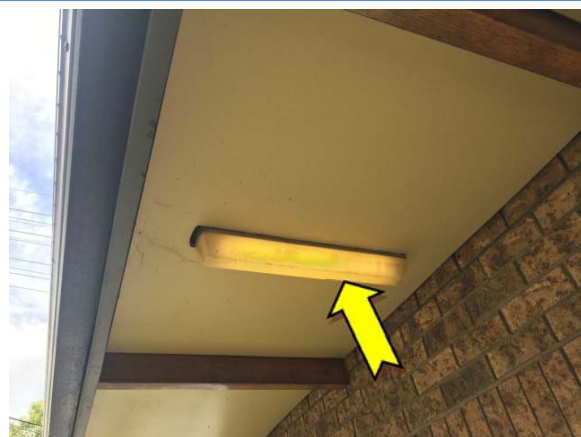
Photo 12. Exterior, north-east elevation, to covered play area, single tubed fluorescent light fittings – suspected PCB-containing capacitors.
