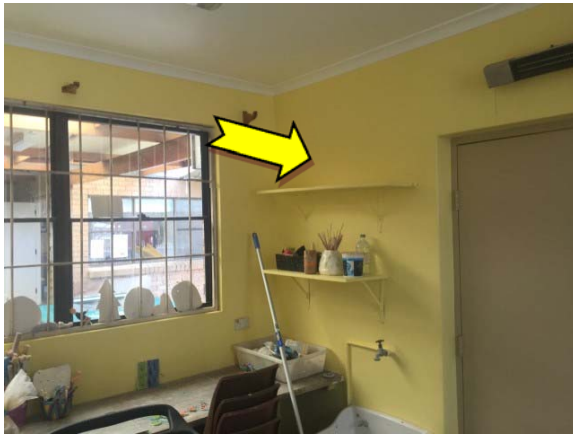
Photo 15. Interior, ceramics room, walls – suspected lead-containing light yellow upper paint systems.
