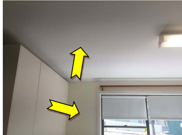
Photo 14. Interior, meeting room, ceiling and walls – suspected lead-containing white and cream upper coloured paint systems.
