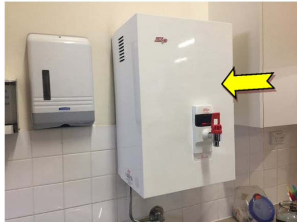
Photo 10. Interior, kitchen, east wall, above sink, hot water boiler – suspected SMF internal insulation material.
