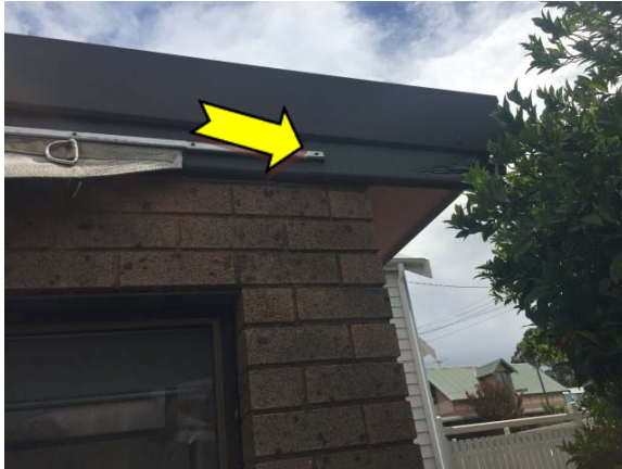
Photo 13. Exterior, throughout, decorative skirting to eaves – suspected lead-containing dark green upper paint systems.
