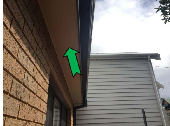
Photo 2. Exterior, north corner, eaves – non asbestos-containing fibre cement sheeting and suspected lead-containing cream upper paint systems.
