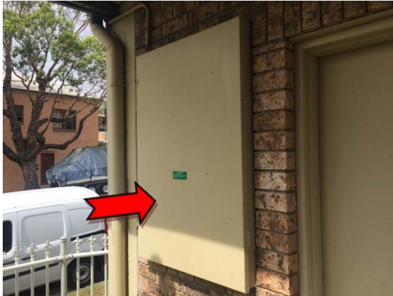
Photo 1. Exterior, north-east elevation, electrical backing board – suspected asbestos-containing bituminous backing board.
